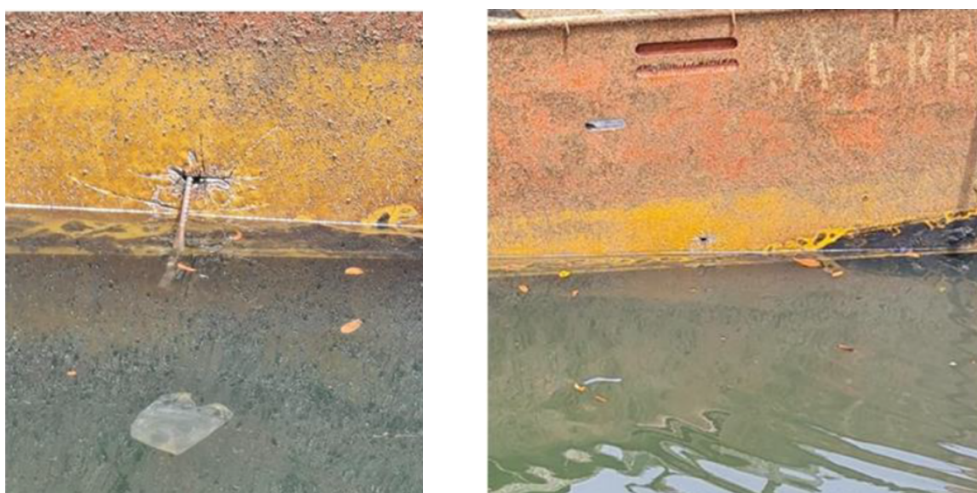
Figure 5: Photographs of the Port Side Hole taken on 5 August 2021. 91
